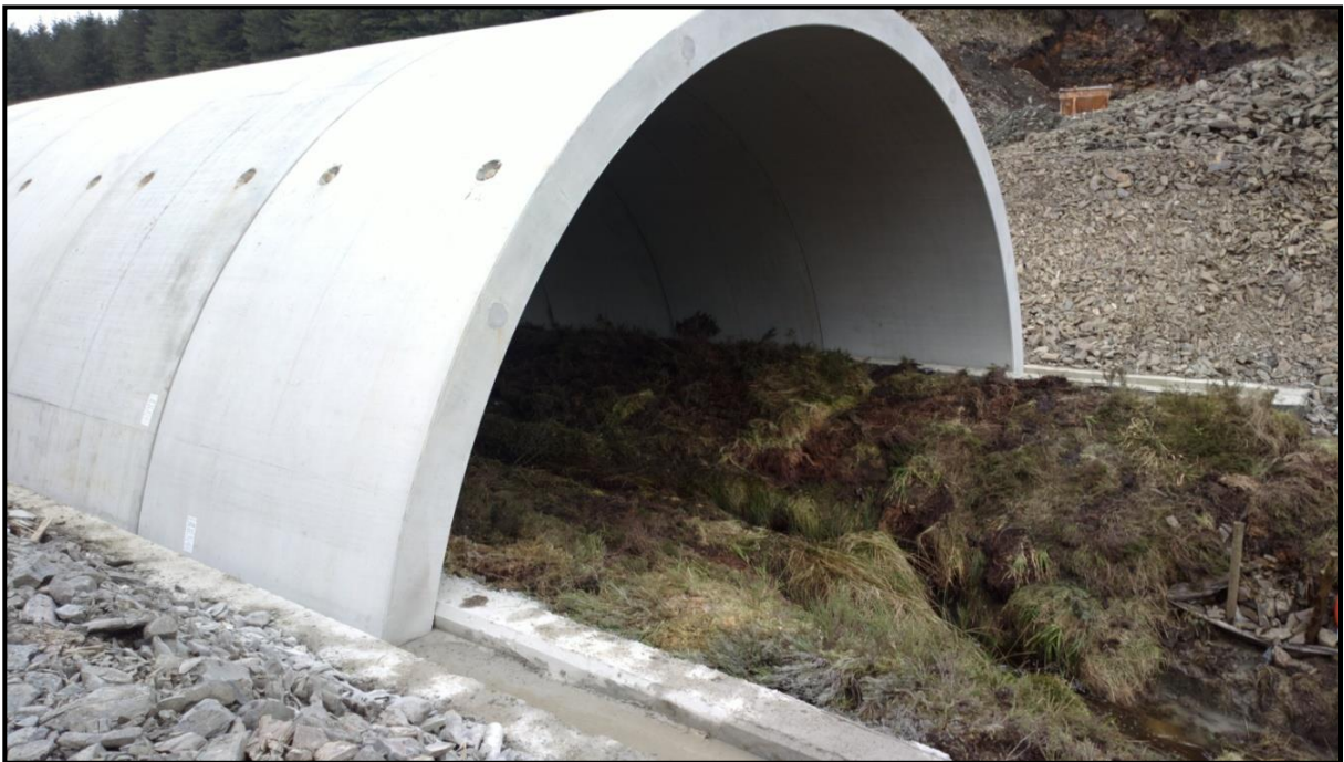
Figure 4.6 Typical clear span pre-cast concrete units in place over an existing watercourse
