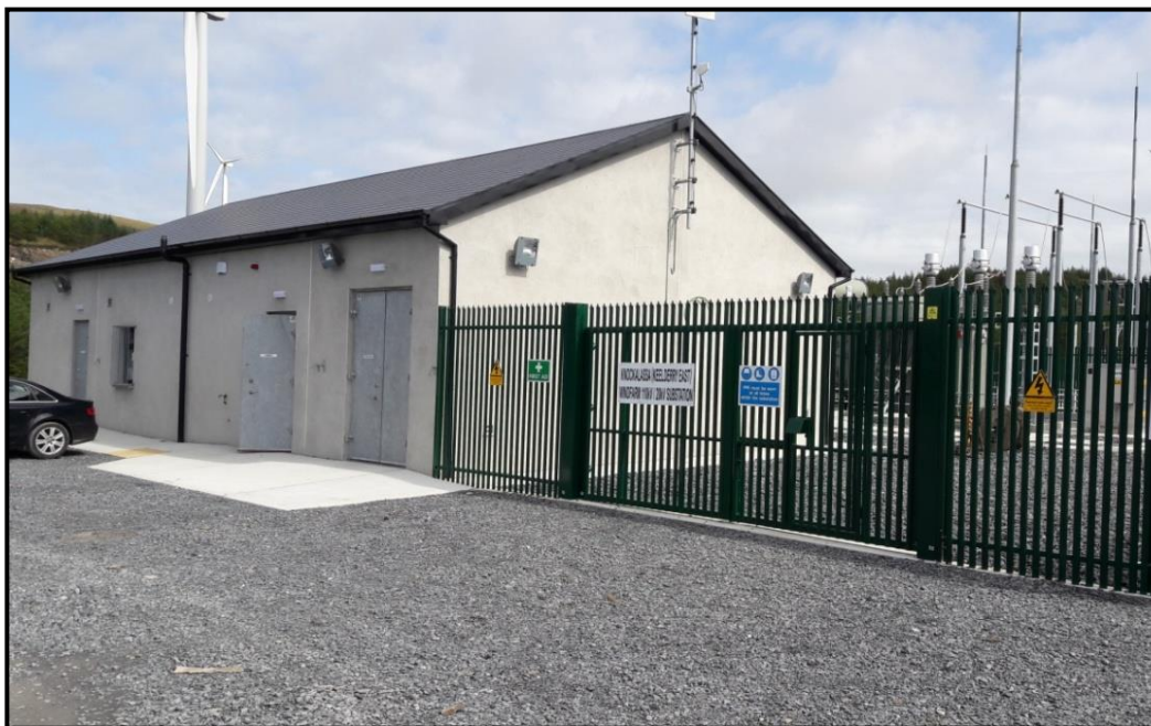
Figure 4.11 Typical substation building and compound
