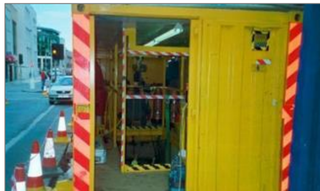
Figure 12 - HV cable jointing container
