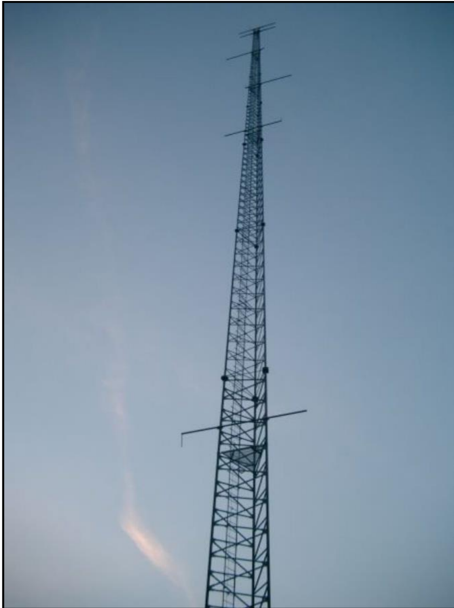
Figure 4.12 Typical meteorological mast on a wind farm
